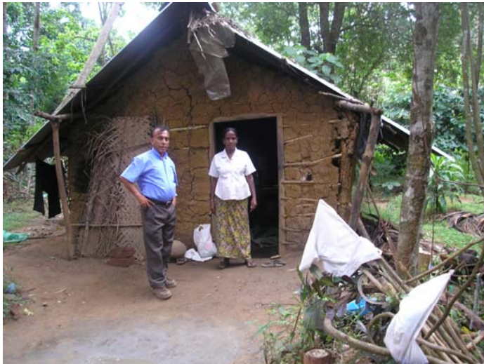
Chandrawathi's old house. The backside of the Roof and the walls have collapsed
